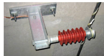
EVA RRA insulator installed in Austrian Blisadona tunnel
