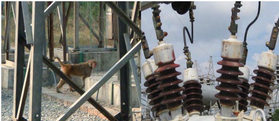
Figure 7. Monkeys in Indian substation and evidence of inter-phase bridging, Greece
