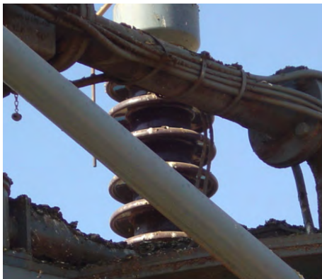
Figure 3. Guano build-up on suspension insulator and on substation equipment.
