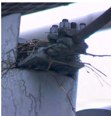
Failure by tracking
