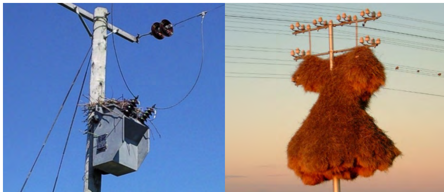
Figure 4. Pole top transformer nest site and huge nest structure in South Africa.
